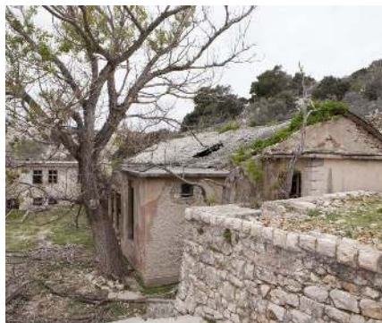
A collapsed stone building.
