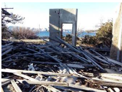
A collapsed roof.
