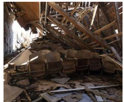
The collapsed interior of a building.
